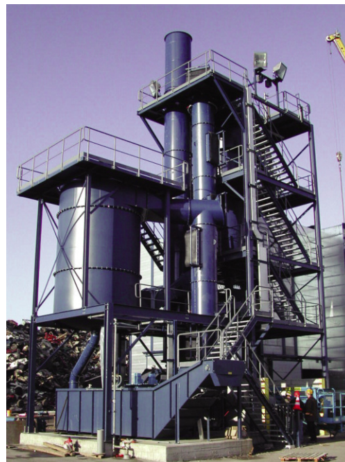
Dust exhausting for 1400 HP-shredder
