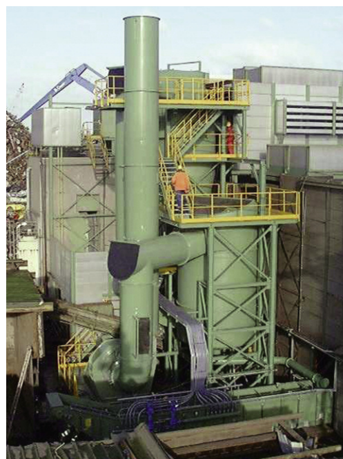
Dust exhausting for 3000 HP-shredder
