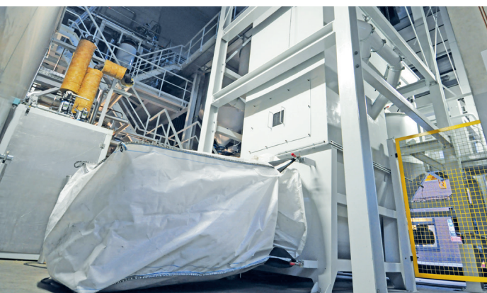
Big Bag compressor in automatic emptying system
