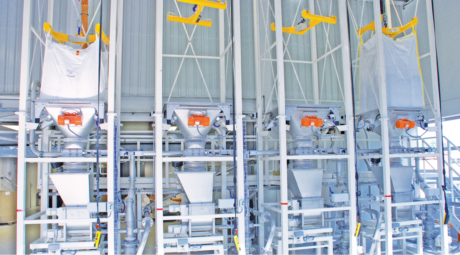
Big Bag emptying stations for the charging of differential metering scales
